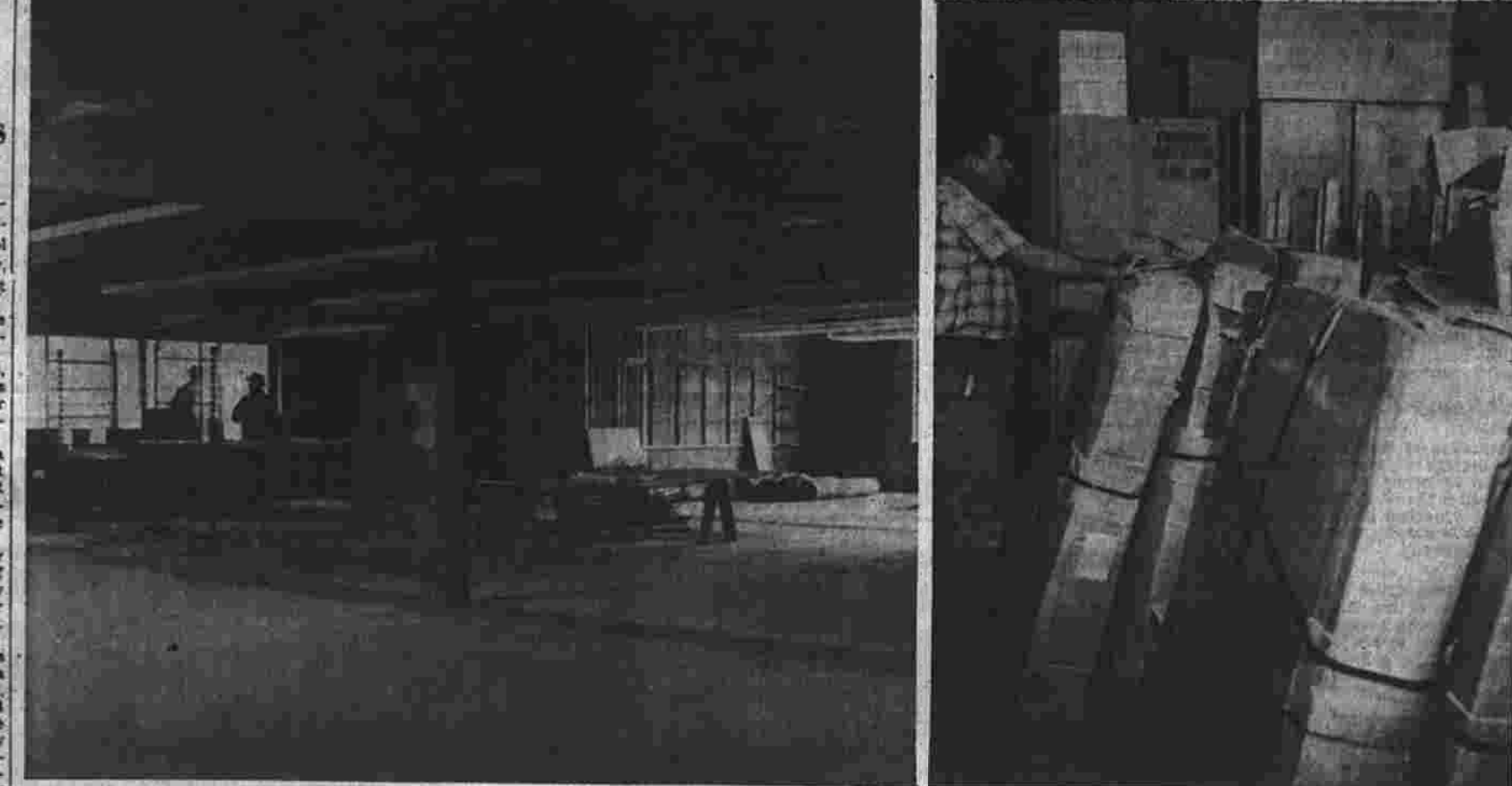
Workers finish one of three senior-wing clusters due to be ready. Equipment stored in Town Hall awaits removal.
